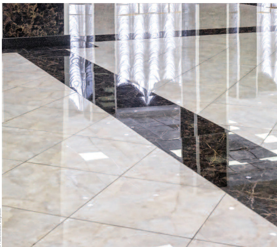
If a floor is shiny, it may appear to be wet or slippery
